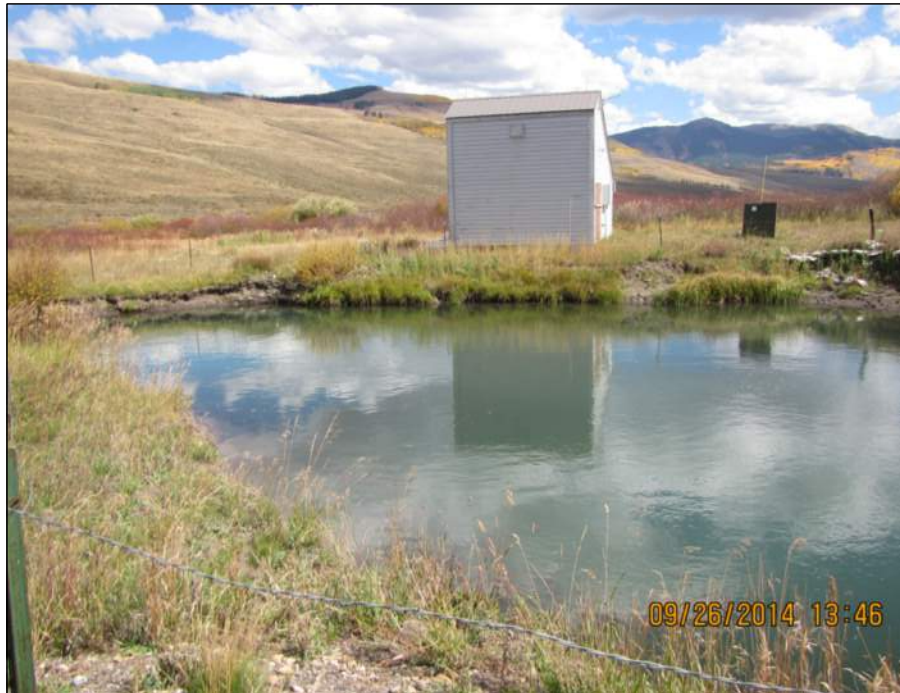
Photograph 1. District pump house and pump forebay/ pre-sedimentation pond.
